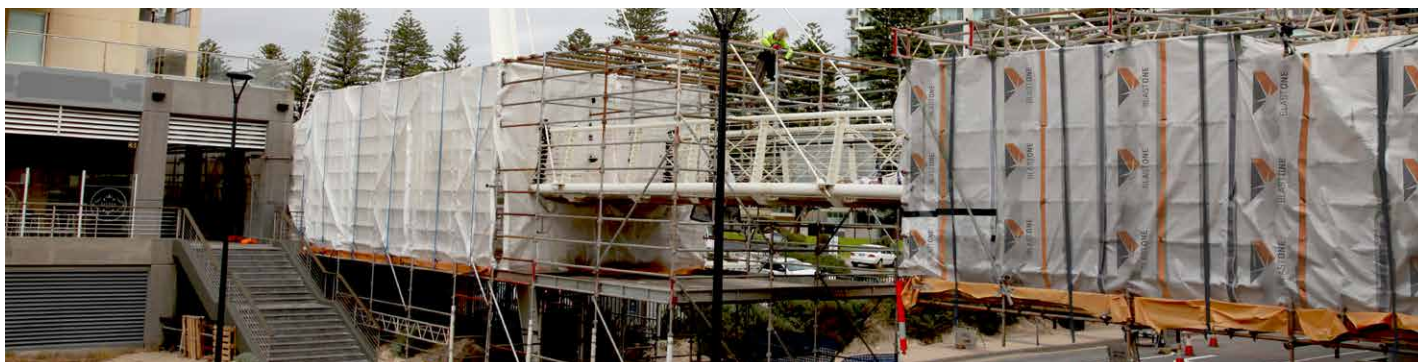
CONTAINMENT SYSTEMS ON THE BEACH-FRONT NEED TO BE BUILT WITH ADDITIONAL STRUCTURAL TIE OFF POINTS SO THE SHEETING IS NOT DAMAGED BY WIND
