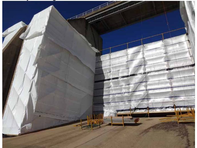
THE USE OF EXTRA WIDE (DOUBLE WIDTH) CONTAINMENT SHEETING ON LARGE VERTICAL CONTAINMENT WALLS ALLOWS FOR FASTER INSTALLATION OF CLADDING
