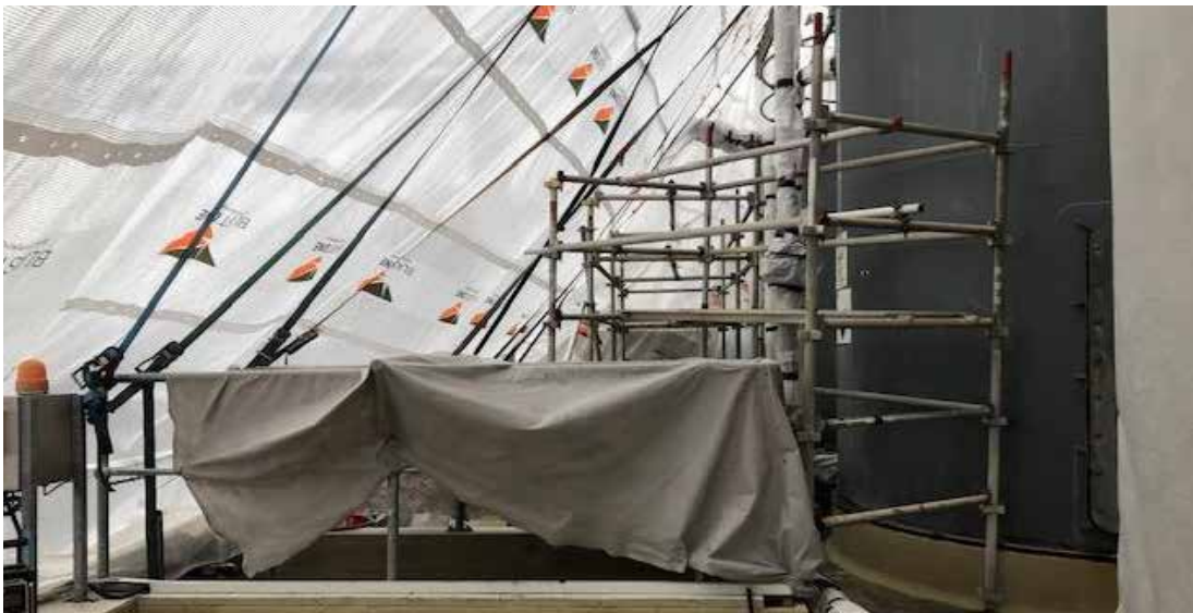
ADDITIONAL MOBILE SCAFFOLDING IS OFTEN NECESSARY INSIDE CONTAINMENT AREAS FOR ACCESS TO SURFACES
