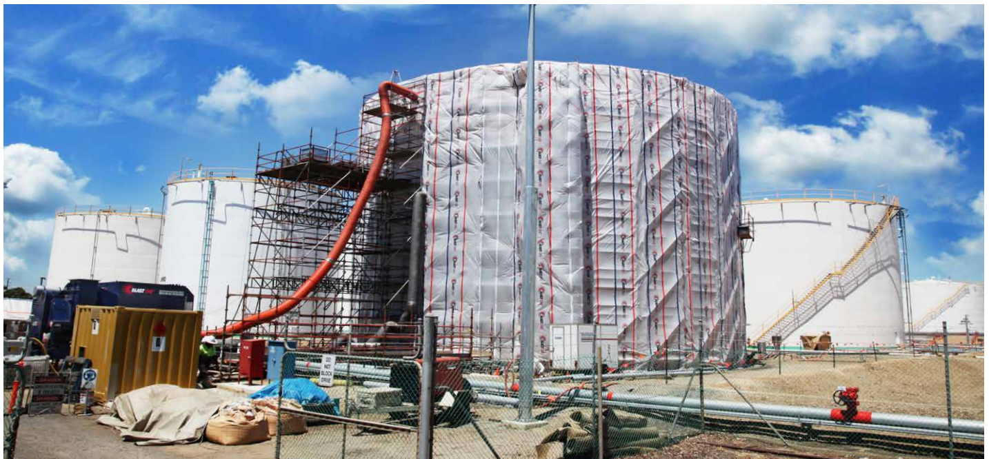
WHILE IT IS EFFICIENT TO CLAD THE ENTIRE CIRCUMFERENCE OF A TANK, IT IS ESSENTIAL TO CREATE "MINI CONTAINMENTS" INSIDE WITH INTERNAL SHEETING WALLS TO REDUCE THE VENTILATED AREA
