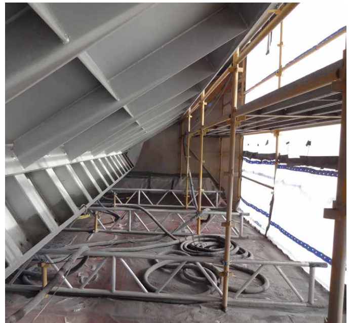
GARNET ABRASIVE ON FLOOR OF CONTAINMENT READY FOR VACUUMING AND RECYCLING. IT IS CRITICAL TO KEEP CONTAINMENT TIGHT FROM RAIN AND WEATHER SO ABRASIVE DOESN'T GET WET
